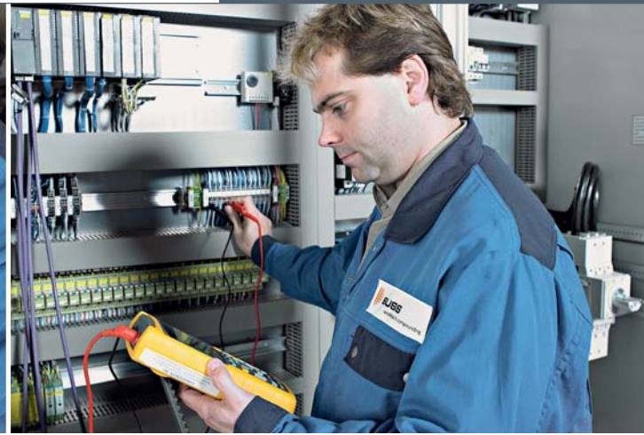
Checking the process control system
